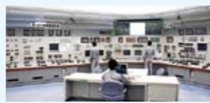
Simulator room at training center of Genkai Nuclear Power Station
