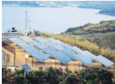
Sakito Photovoltaic Power Plant
