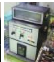
Control system for inrush current of transformer
