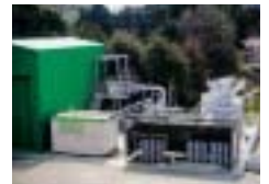
Wood biomass gasification facility
