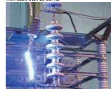
KO horn (arc horn for 66kV transmission lines)
