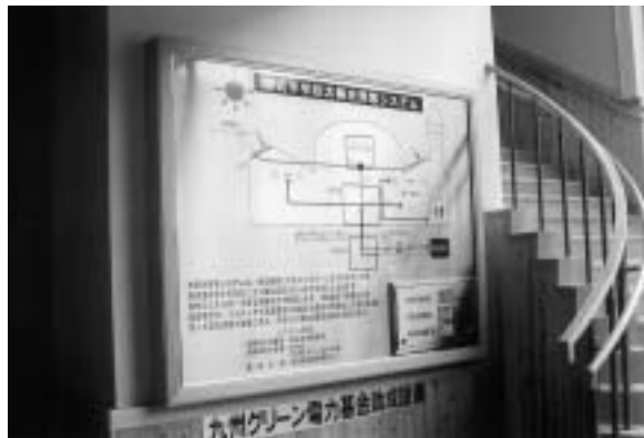
Photovoltaic power generation monitoring panel Neijme Junior High School (Kagoshima Pref.)
