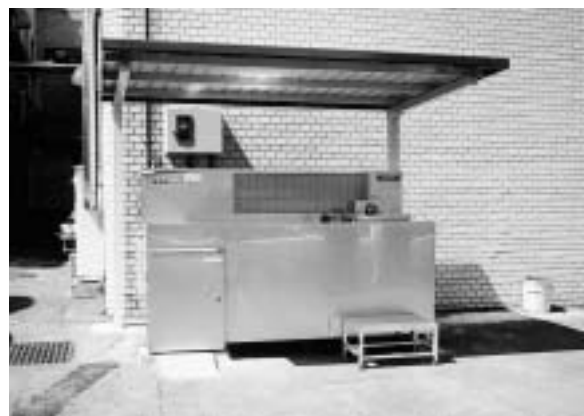
Composting facility on trial at Education & Training Center
