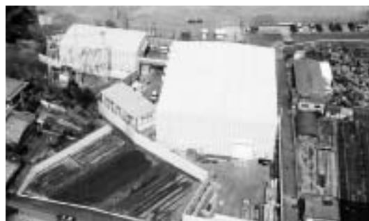
Tunneling work, part of the new construction of a Kurume branch-line (start shaft side)
