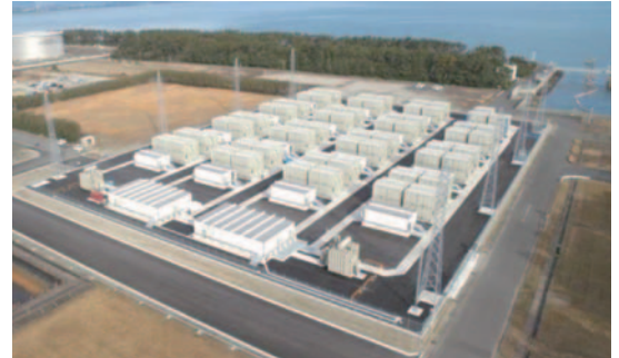
Aerial view of the Buzen Accumulator Substation
