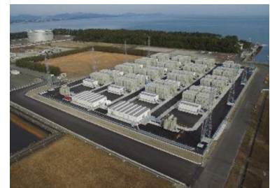
Buzen Battery Storage and Transformer Station
