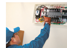
Inspection of distribution boards
