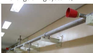
Automatic fire extinguishing system (halon fire extinguishing systems)
