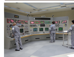
Operation using a simulator
