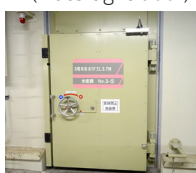
Water overflow countermeasures (watertight door)
