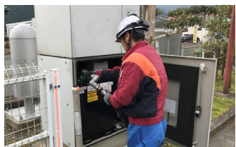
Fuel supply support for monitoring post
