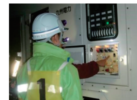
Power supply by high-voltage generator truck (nighttime)
