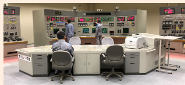
Simulator room at the Genkai Nuclear Power Station Training Center
