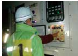
Power supply by high-voltage generator truck (nighttime)
