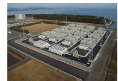
Buzen Battery Storage and Transformer Station
