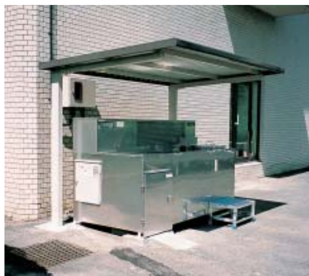
Composting facility installed at Education & Training Center
