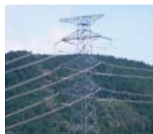
Normal steel tower (unpainted)
