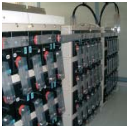
(LL lead storage battery)
