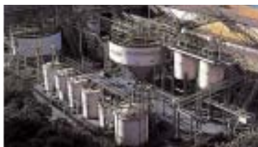
(Comprehensive wastewater treatment facility)
