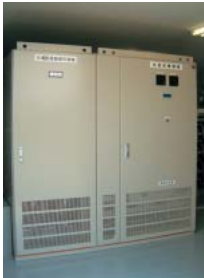
(Bidirectional converter and system interconnection protective board)
