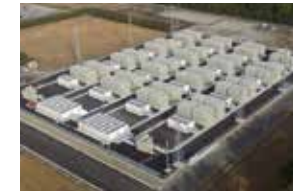
Buzen Battery Storage and Transformer Station
