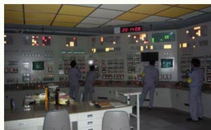
Drill conducted under total AC power blackout
