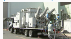
Practice drill on supplying power using mobile equipment
