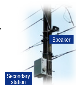
System installed on a utility pole
