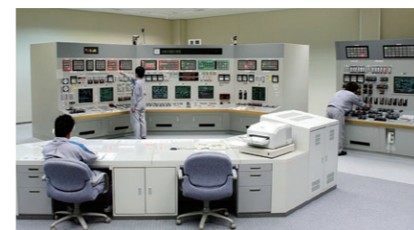
Simulator room (for units 3 and 4)
