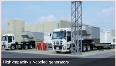
High-capacity air-cooled generators
