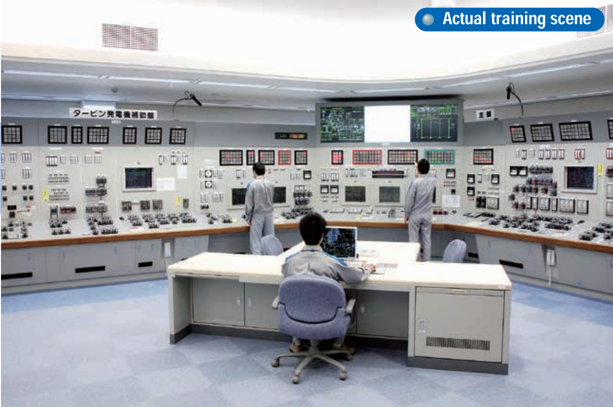
Simulator room (2-loop operation)
